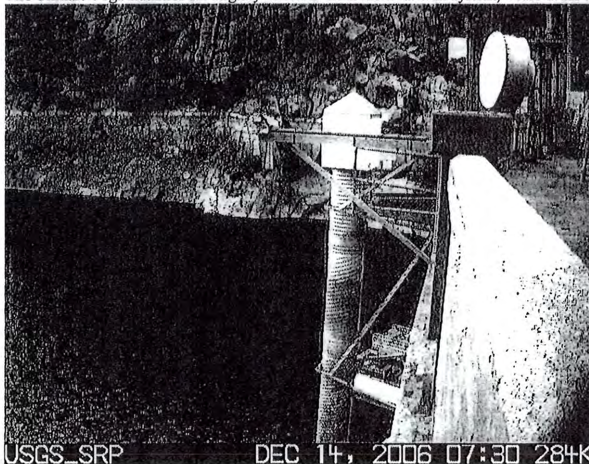
Figure 2. Photo of installed radars and stilling well at Horse Mesa Dam, Arizona.
