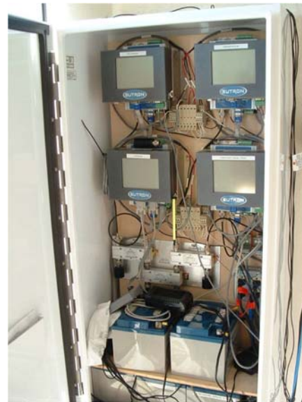
Figure 6. Four DCPs and batteries in metal enclosure at field site.
